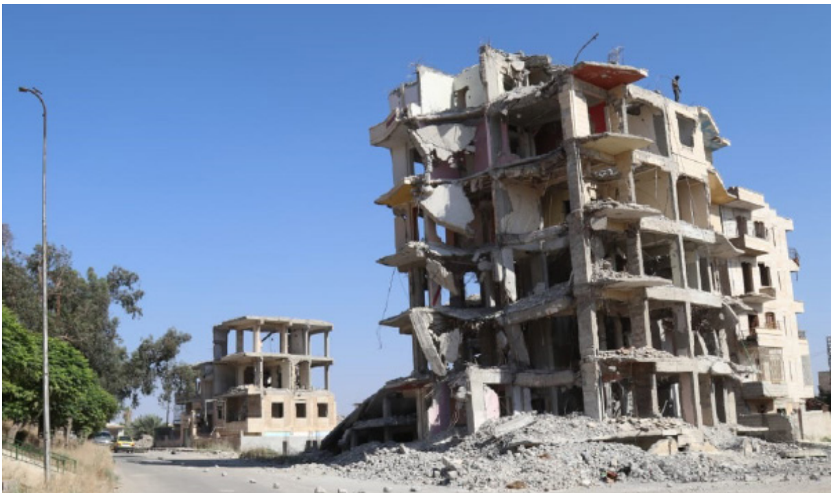
Destroyed buildings in Raqqa city four years after the city was recaptured from ISIS. Photo taken on 1 June 2021/ Save the Children
